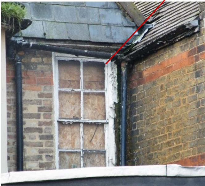
One of the worst windows.
