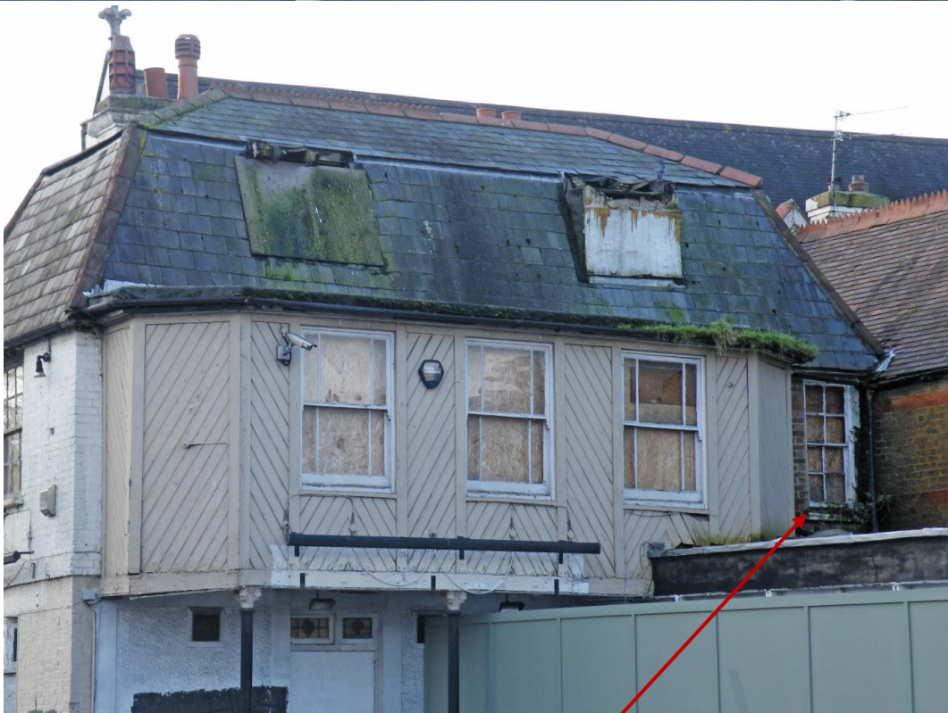
Blocked gutters and rotting timber. Rainwater is almost certainly running through the building.
